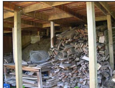
If items stored under the deck can ignite from embers, deck and structure will follow along. Don't store combustibles under decks!
