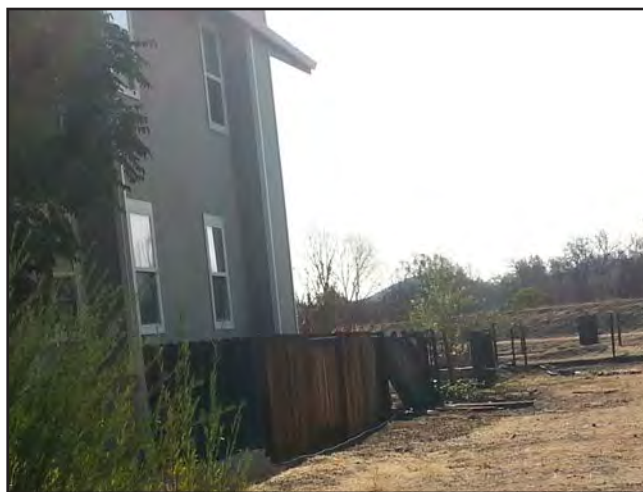
Create non-combustible space between the wood fence and the house walls with metal gates, and similar material. This fence would have burned to the house walls had firefighters not arrived to extinguish the fire.
