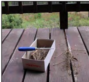
Keep needles and debris from accumulating between deck boards or between deck and siding.
