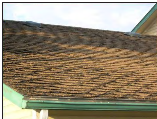
Though it may have originally had a Class A rating, this old, weathered asphalt composition shingle roof would no longer provide adequate protection against embers and heat.
