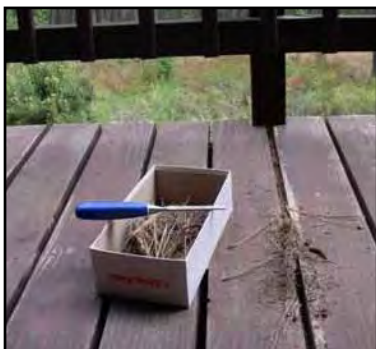
Keep needles and debris from accumulating between deck boards or between deck and siding.
