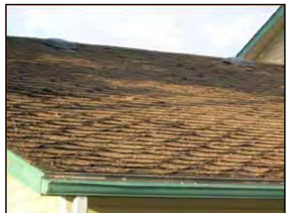
Though it may have originally had a Class A rating, this old, weathered asphalt composition shingle roof would no longer provide adequate protection against embers and heat.
