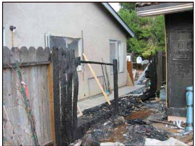
Create non-combustible space between the wood fence and the house walls with metal gates, and similar material.
