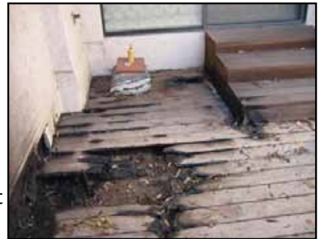
Consider replacing ground level wooden decks with non-combustible patio materials such as brick, stone or concrete.
